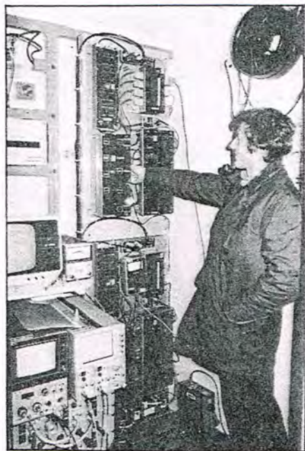
Inside Hedleyhope. Gordon Bowhay, of the BBC's transmitter capital projects department, is putting the finishing touches to his 'Blue Streak' installation. The instruments at bottom left are test gear, not station equipment.
